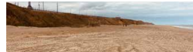
Significant sandscaping work has been undertaken to secure the land in front of the Bacton Gas Terminal
